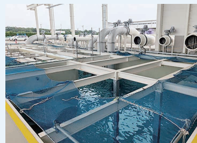
Ono Plant large pump operation inspection equipment (supports pumps up to 1,200 mm in bore)
