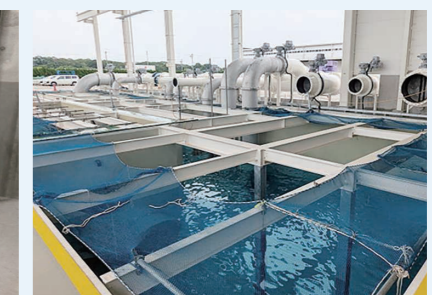
Ono Plant large pump operation inspection equipment (supports pumps up to 1,200 mm in bore)
