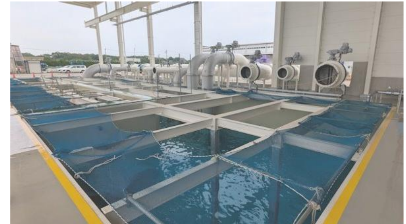
Ono Plant large-scale pump operation inspection equipment (works with pumps up to 1200 mm in diameter)
