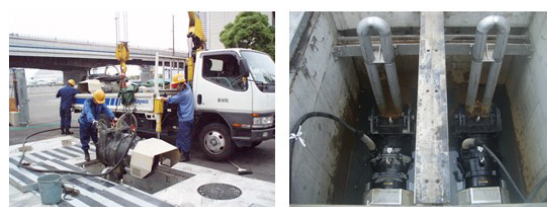
K City Rainwater drainage pumps (horizontal axial-flow)
