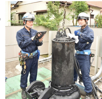
ShinMaywa Aqua Technology Service, Ltd. is responsible for maintenance
