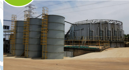
Wastewater treatment equipment (Wuhan, China)
