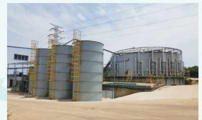
Wastewater treatment facilities (Wuhan, China) by ShinMaywa (Chongqing) Environmental Solutions Co., Ltd.
