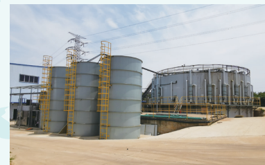
Wastewater treatment facilities (Wuhan, China) by ShinMaywa (Chongqing) Environmental Solutions Co., Ltd.
